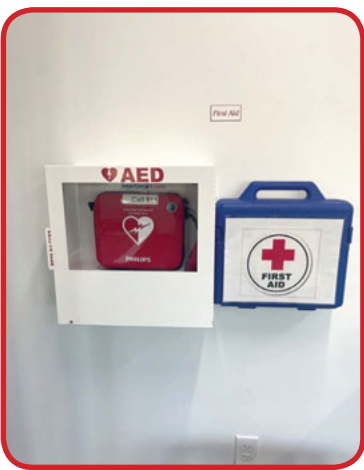
This AED is located in the Exercise Room off the Pool.
