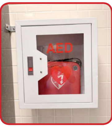
This AED in the Craft Building has been moved right inside the door of the men's room by the Tennis Courts.
